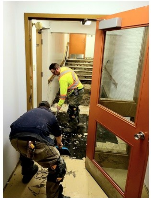
An installation team from Curtis Carpets works on re-tiling the rain-damaged lower-level foyer of our parish centre. This completes the work...
