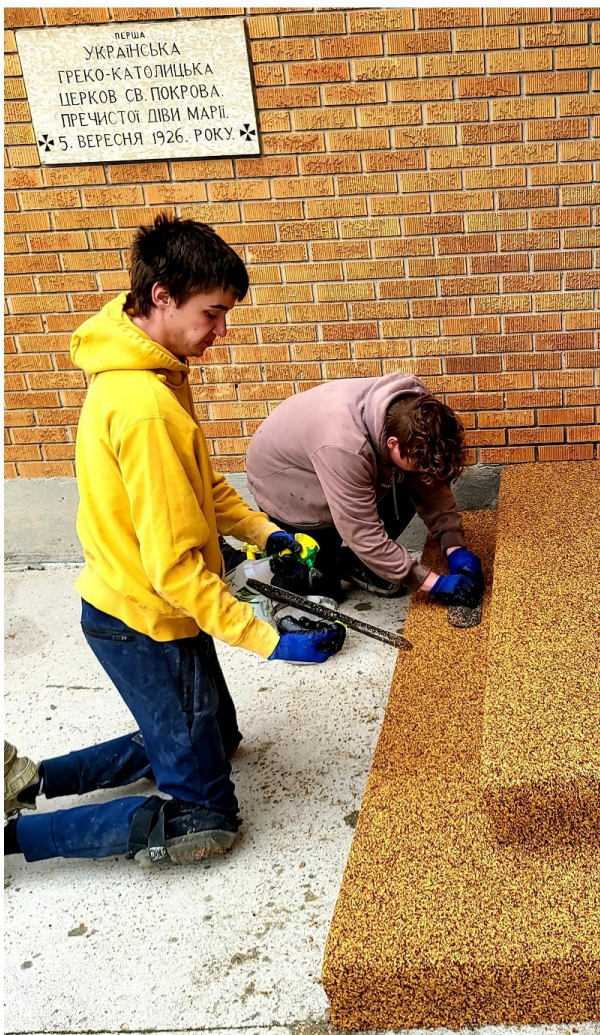
Lookin' pretty classy! Seth and Jer of Jerry's Concrete Works. put the finishing touches on our new Centenary Church Steps!
